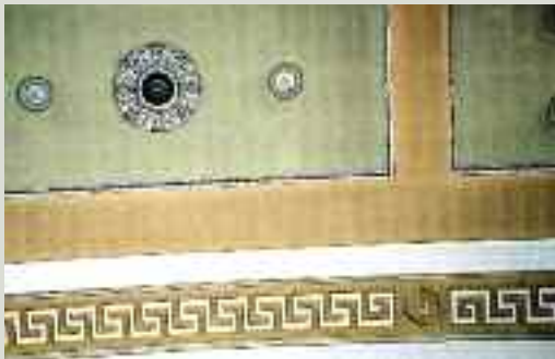
This plastered ceiling has no insulation above it. Discolouration can be seen on the plasterwork between the timber joists located above, as the timber is slower to transfer heat to the cold roof space than the plaster alone. Dust particles in the warm air passing through the plaster remain trapped on the surface causing the discolouration
