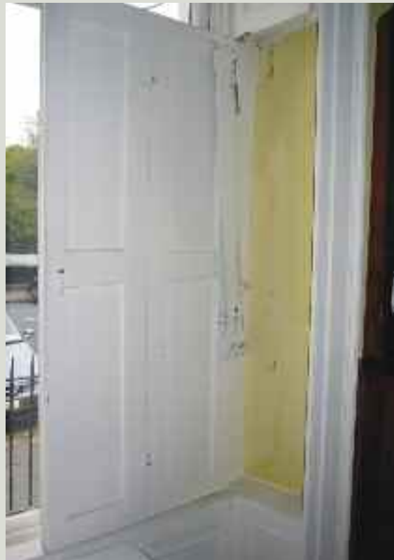
A well-sealed shutter lining
