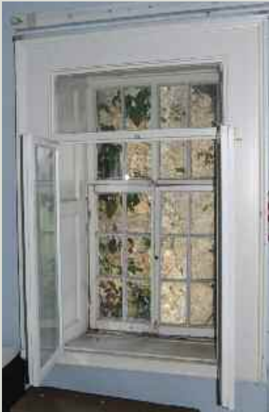
An Edwardian window with 1950s secondary glazing. The secondary glazing is chunky and does not match the original window profile and blocks light from the room. The position of the frame within the opening prevents the shutters from being used
