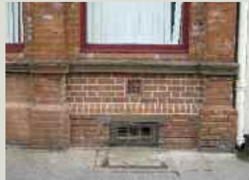
A floor vent to ventilate the ground floor was built into the wall between the cellar and ground floor windows as part of the original design
