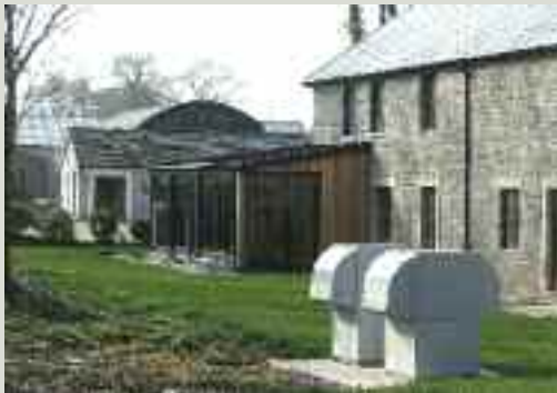
Air-to-water heat exchangers: a heating system provided to a converted stable building. The grey metal casing will be camouflaged by future planting
